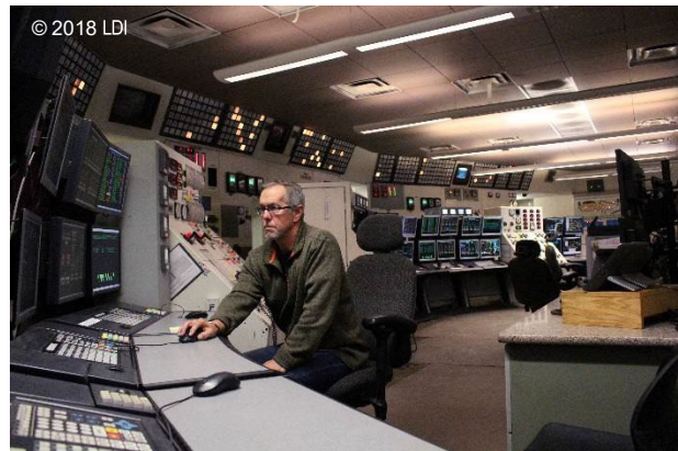
Figure 11. Control Room at Naughton Power Plant.
